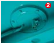
Fuel drain valve
