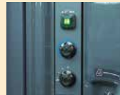
Air conditioner switch
